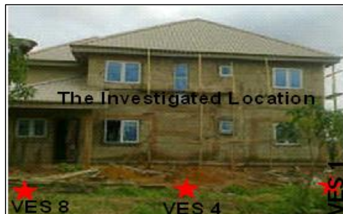
Figure 30: Location of the VES stations and the patched cracks in the building.
