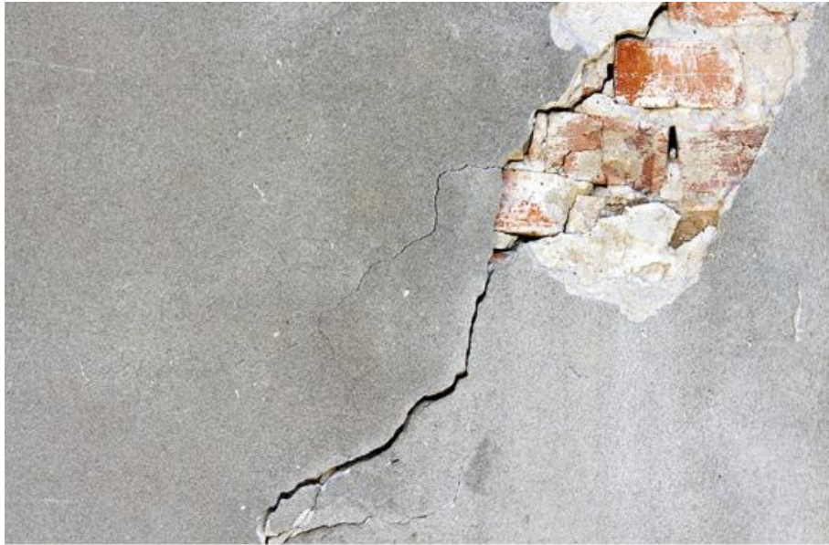
Figure 28: Differential settlement in wall column as a result of subsurface structures (faults)
