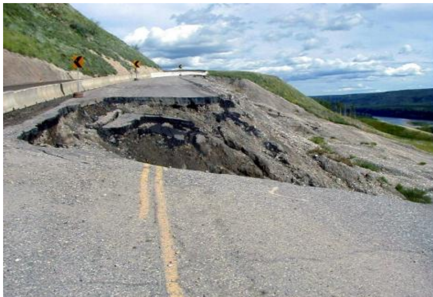
Figure 29: Road failure as a result of geologic fault
