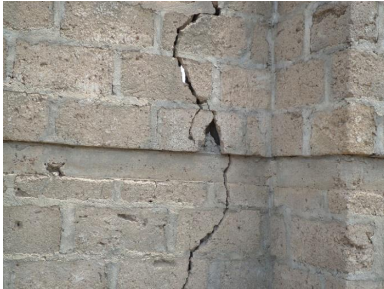
Figure 31: The cracks noticed at the Eastern fence that separates the building from another house.
