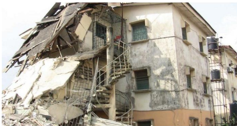
Figure 27: Building collapse in Lagos as a result of subsurface incompetency
