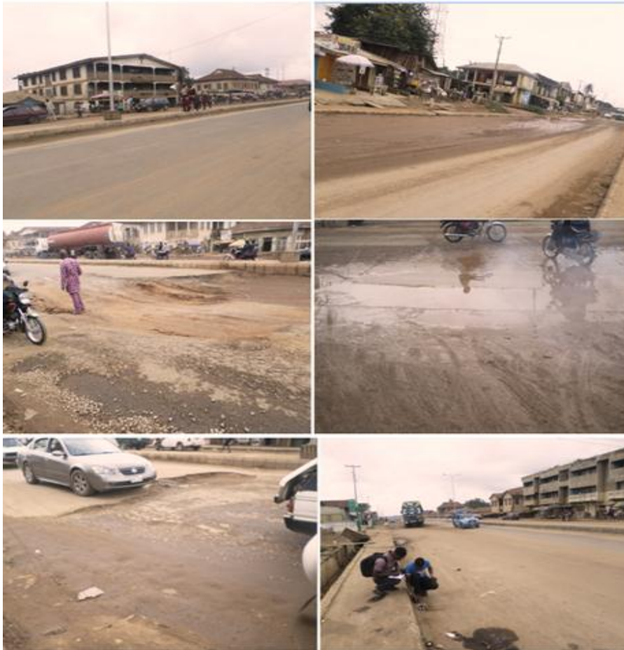
Figure 38: Snapshot of some stable and deteriorated portion of the area
